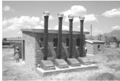
An "enviroloo" (dry composting toilets) mandated by the Department of Public Works in the Northern Province of the Republic of South Africa (2002)
